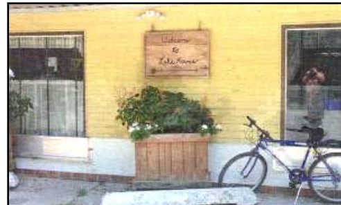
Figure 28 - This home in Jefferson Parish, LA has permanent shields sealing the space under the windows
