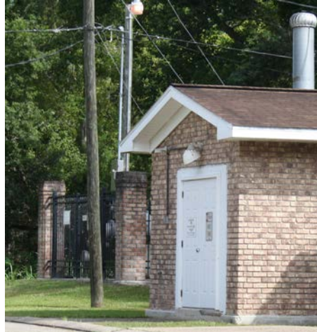
Figure 8 - Sanitary System Pump in Westview Drive Study Area
