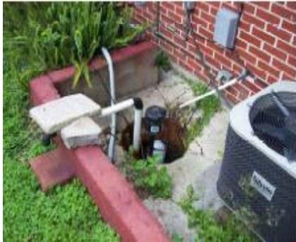
Figure 20 - Water collects in this basin, or sump, and is pumped out by a sump pump.
